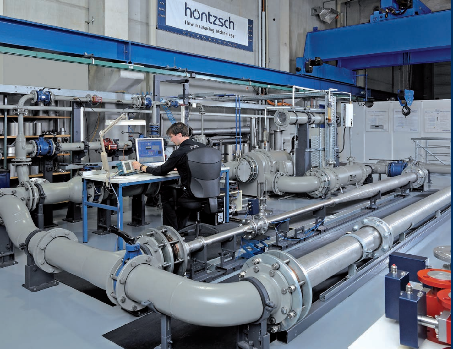
Volume flow calibration installation, pressure up to 10 bar, 1 MPa, nominal value up to DN200
